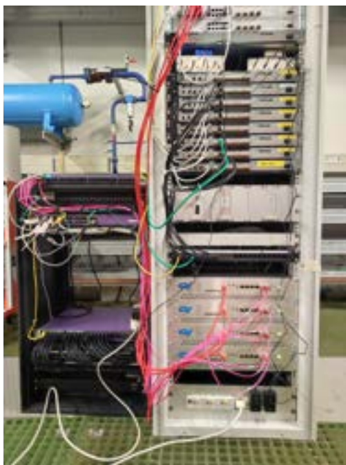
Figure 3: Digital units in Elettra service area.
