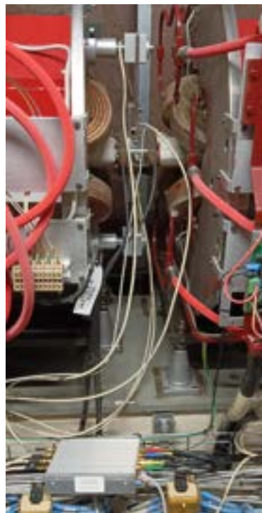
Figure 1: PTFEs in Elettra tunnel connected to BPM pick-ups.
