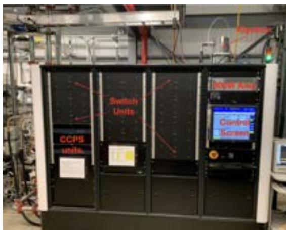
Figure 2: The first K400 modulator being tested in the utility shed with the Canon E3712 Klystron. There are two CCPS units and twelve IGBT switch units in the system.
