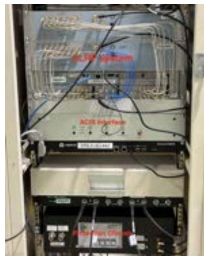
Figure 3: The Libera LLRF Systems are installed in the LLRF rack, with the new ACIS interface and protection chassis connected.
